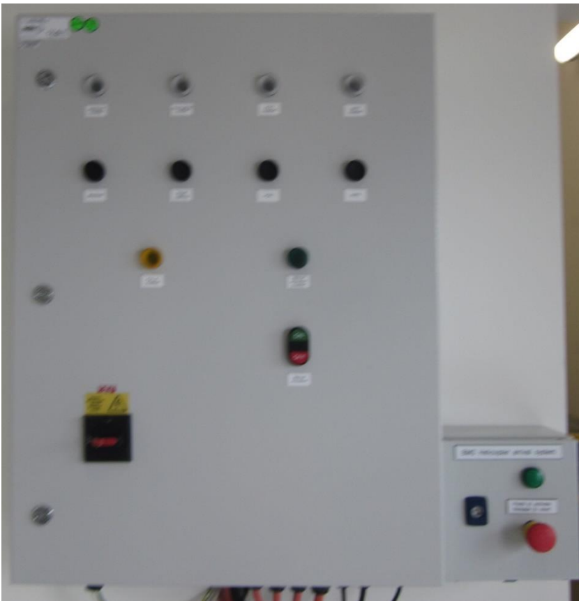
Figure 8 – Heliport Lift Lobby Equipment – Northern Wall – Heliport Lighting Control Panel
