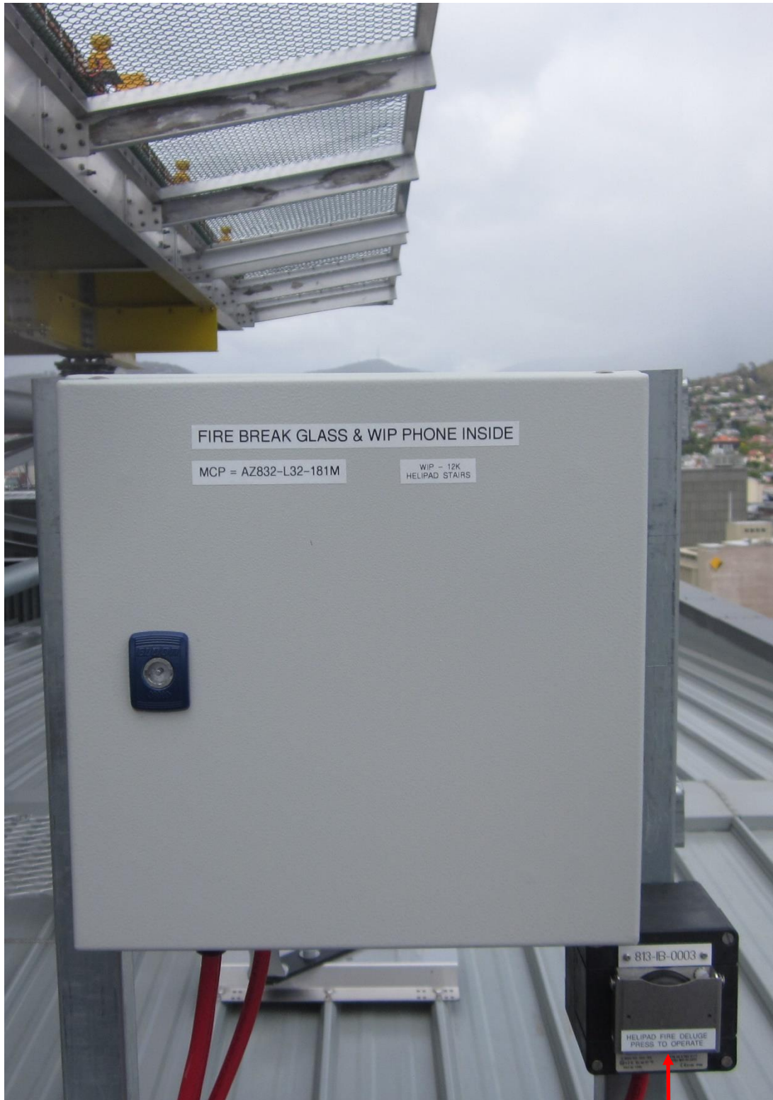
Figure 15 – Heliport Emergency Evacuation Stairs – Second Landing – Break Glass Alarm, WIP Phone and DIFFS Activation Button
